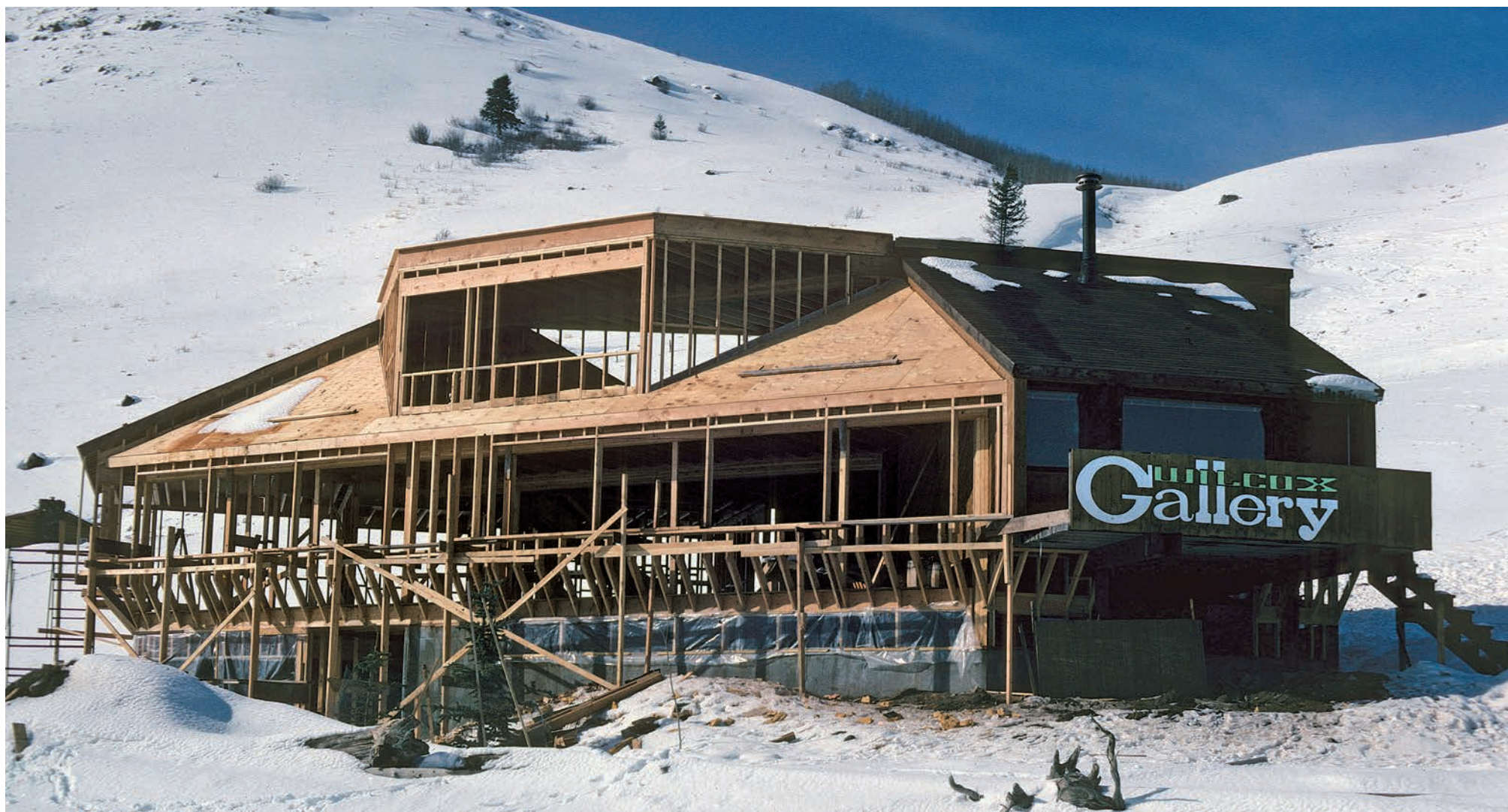
The main Wilcox Gallery addition in construction phase in 1978. The stairs on the porch no longer exist, though at one time they provided the only access to the building.
